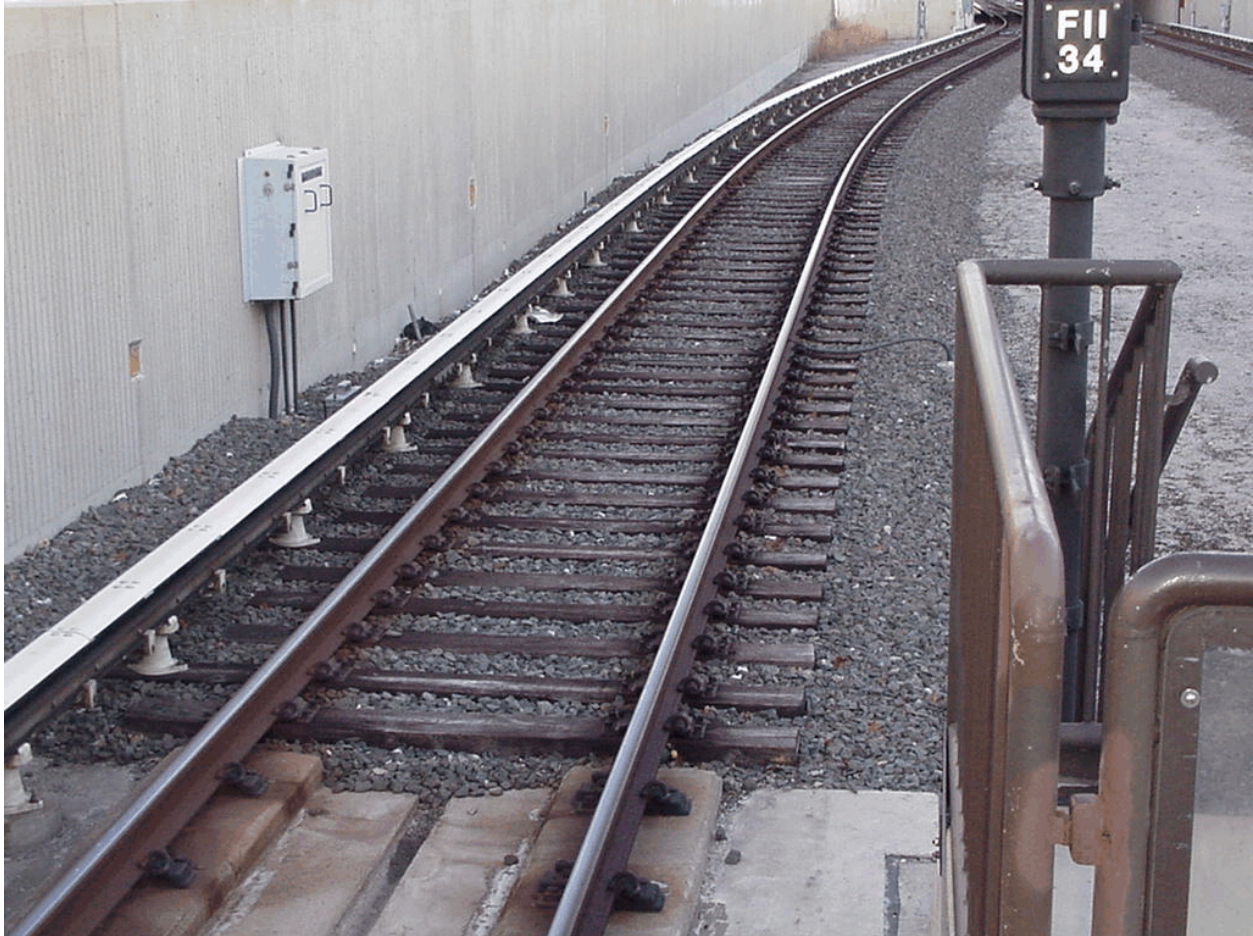
Ballasted Track, Branch Avenue Station
